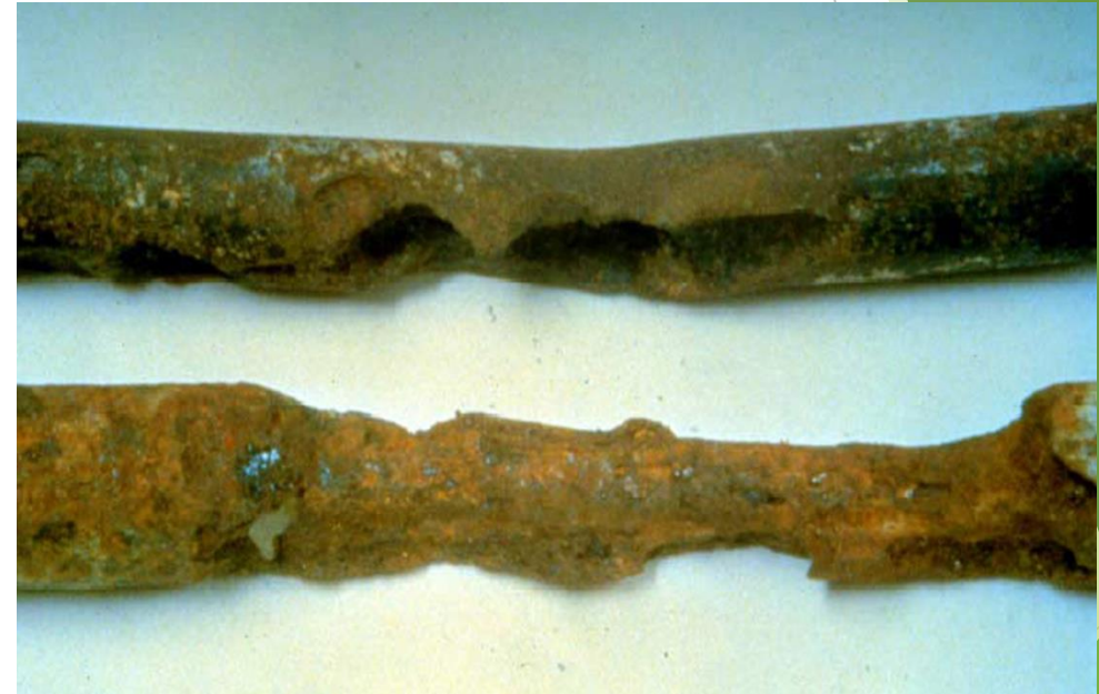
Examples of pitting corrosion induced by chloride ingress after 5 years
